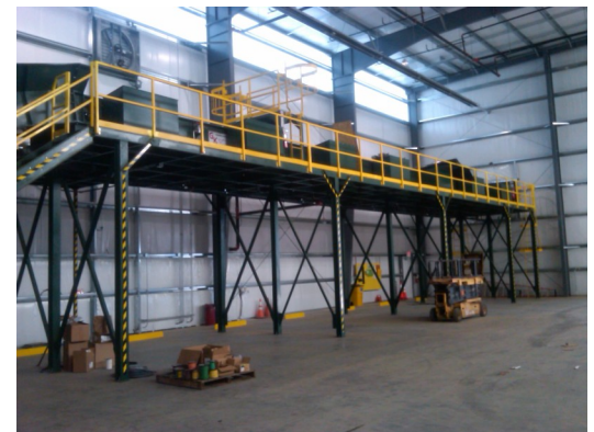
Items are separated and dropped into containers or dump trucks parked below.
